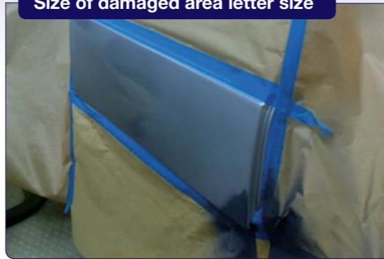
Size of damaged area letter size
